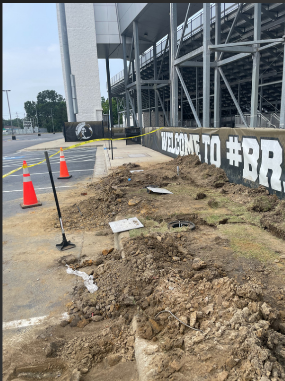
EV Charging Station
