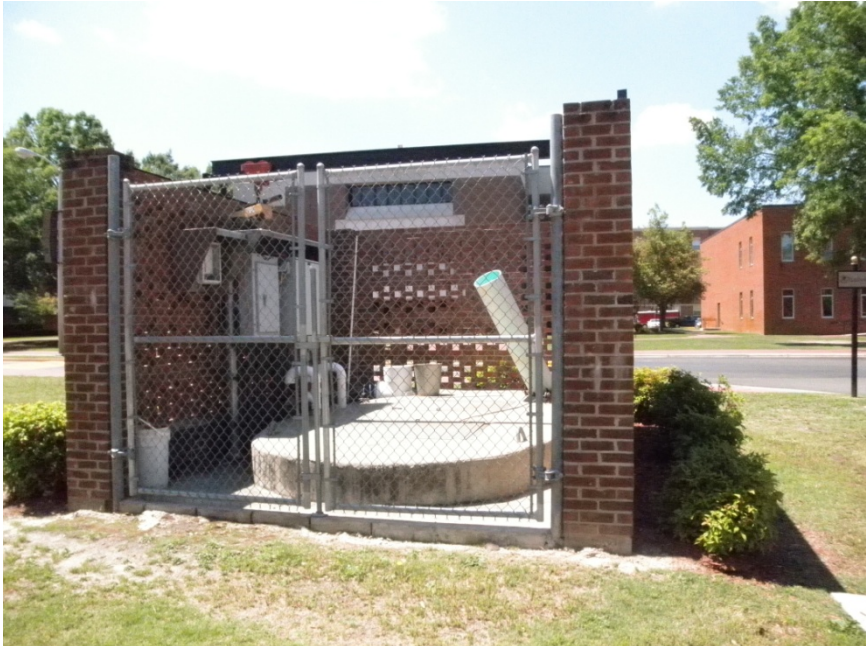
Lift station at NW corner needs to be disguised/relocated with D.F.Lowry renovations or with Information Commons.
